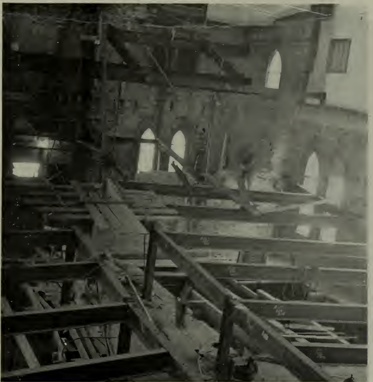
The steel is in place for the Pickard Theater in Memorial Hall
